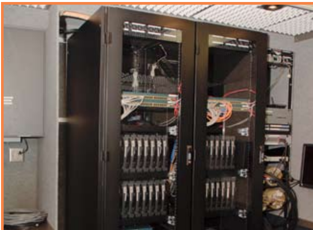
The Liebert Foundation MCR (Mini-Computer Room) features load-sized, computer-grade air conditioning which delivers cool air to sensitive equipment on all levels.
