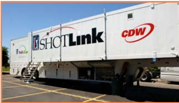
CDW recently completed improvements on two of the ShotLink trailers’ rack and cooling systems, as well as enhancing cable management and power distribution.
