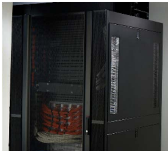
Installed on AR3340 enclosure
